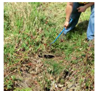
Roadside ditch in need of maintenance. Vegetation is blocking inlet to pipe.
