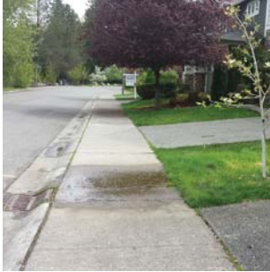
Example of groundwater seepage
