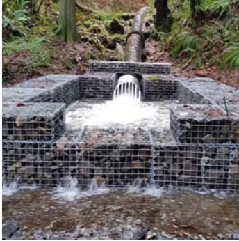
Evans Creek HDPE pipe outfall energy dissipation
