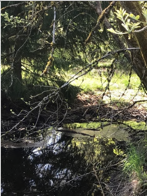
Photo 2. Stream is ponded downstream of 244 th Avenue SE culvert.
